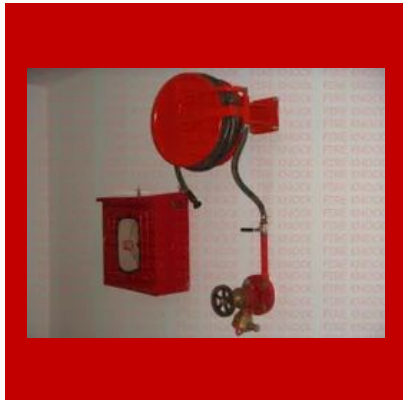
Fire Hydrant System
