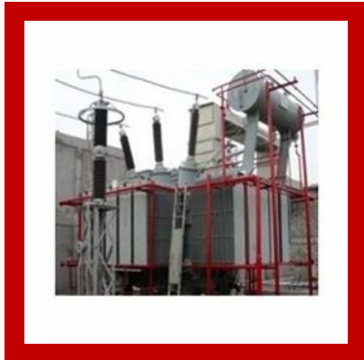
High Velocity Water Spray System
