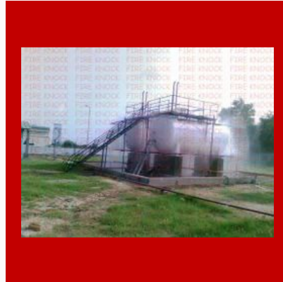
Medium Velocity Water Spray System
